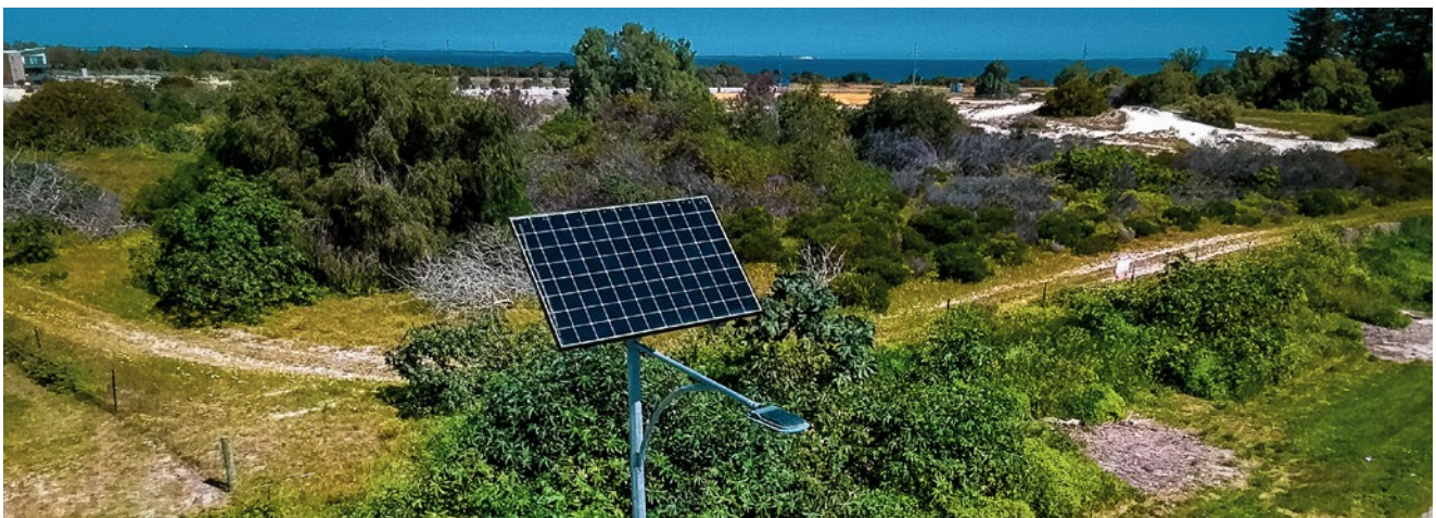
Image 5: Solar powered LED light, Rollinson Road, North Coogee
