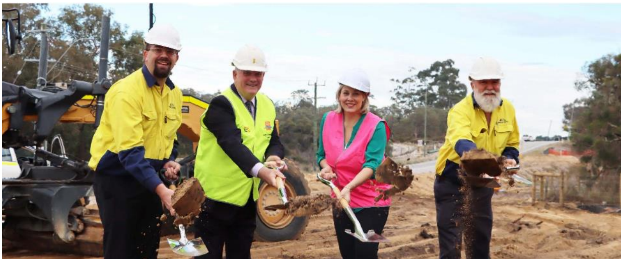
Photo: (from Left to Right) General Manager Tracc Civil Pty Ltd Frank Janssen, Mayor Howlett, Deputy Mayor Lara Kirkwood, Operations Manager Tracc Civil Pty Ltd Craig Risbey at Jandakot Road Stage 2 sod-turning - May 2021
